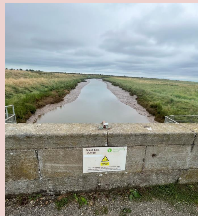
Great Eau Tidal Outfall (photograph by Arup)
